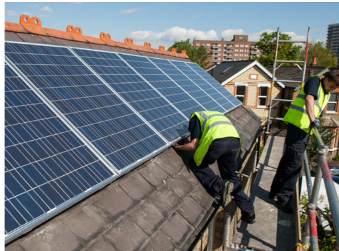
Figure 11 Solar Panel installations
